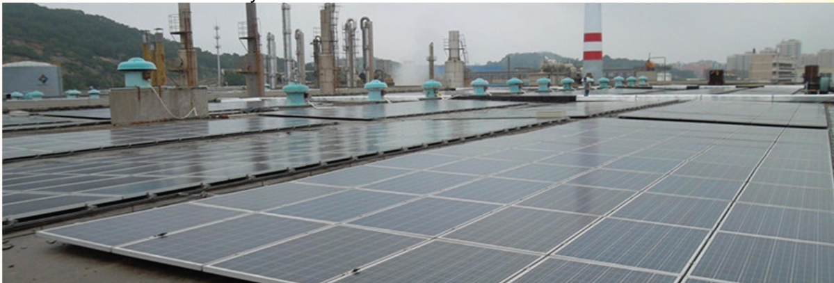
Photovoltaic Power Generation System
